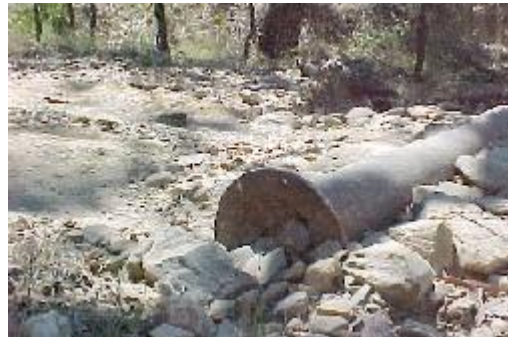
Hazardous state of causeway towards Abbott's Ln
